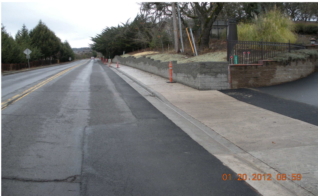
(Above) – Completed sidewalk and retaining wall within the Hillcrest Sidewalk Improvement Project.
